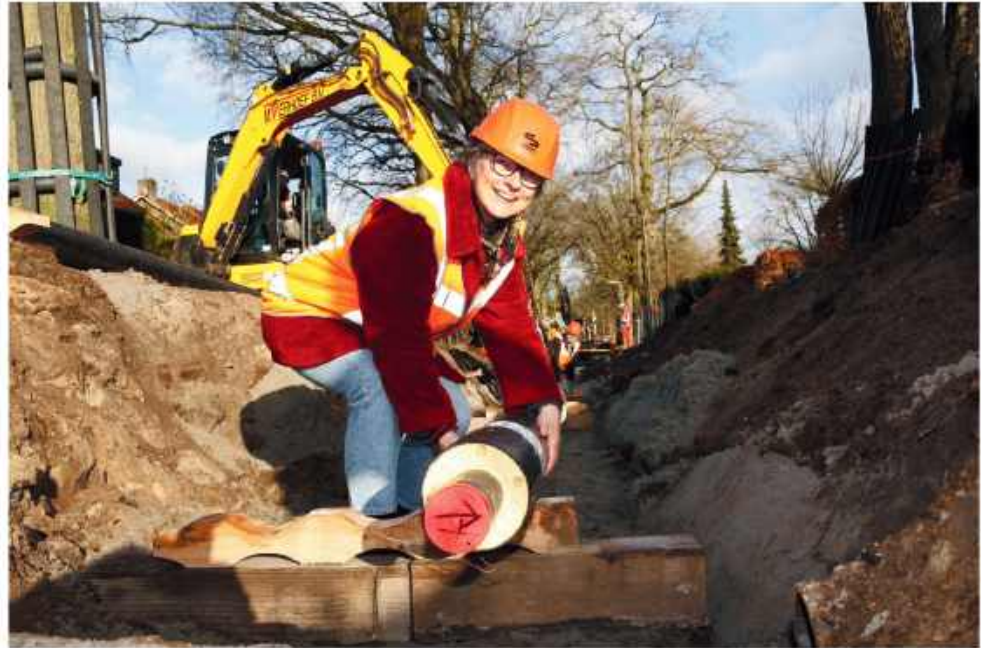
Alderman for sustainability of Gooise Meren places the first pipeline of the citizen-led project @ Wattnu energy community
