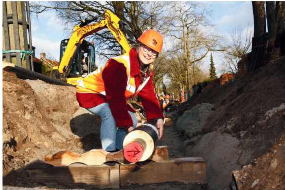
Alderman for sustainability of Gooise Meren places the first pipeline of the citizen-led project @ Wattnu energy community
